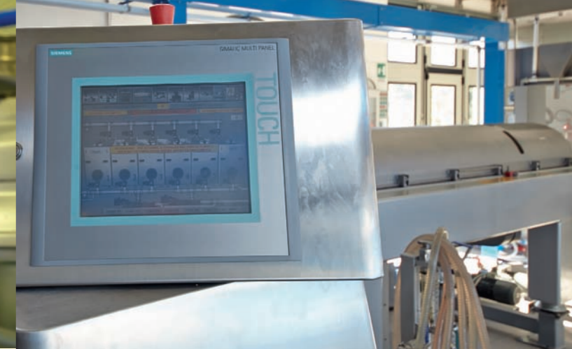
Automation and control
